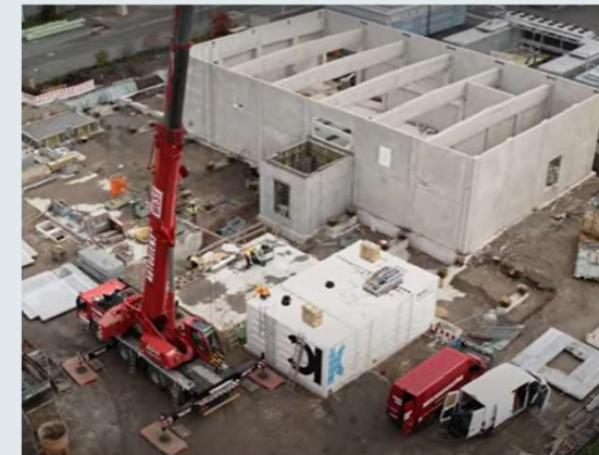
INERATEC plant at IPH (operational Dec. 24)
